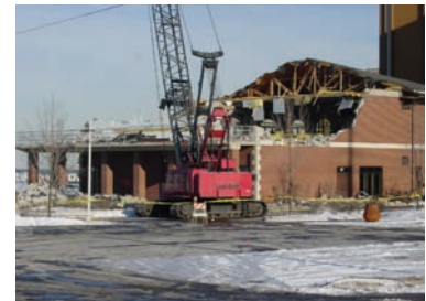
Pictured top left: Hammond Marina under construction last June. Above: The old Hammond Yacht Club demolished.
