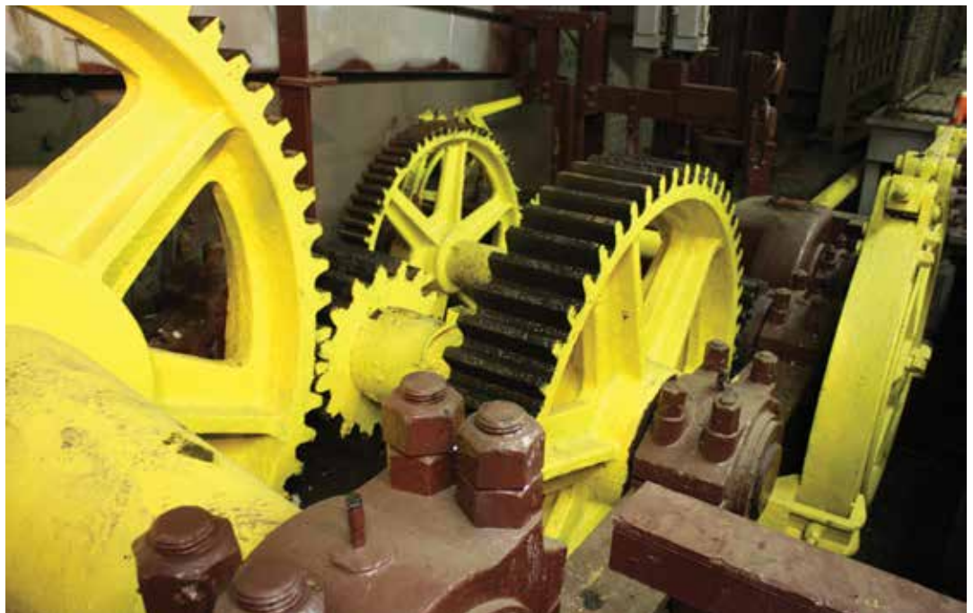
Operated by a motor of only 108 horse-power, the bridge gears barely make a sound as they open the massive bridge.
